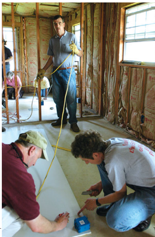
Vermont Bishop Thomas Ely, Albany Bishop William Love and Presiding Bishop Katharine Jefferts Schori worked on hanging sheetrock in a Gulport, Mississippi house.
